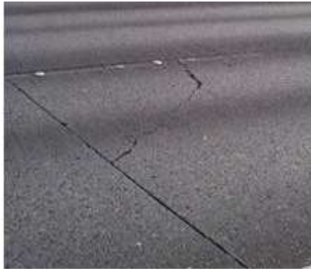
Figura 2.10 – Rotura de canto (Pavement Interactive ©2016)
